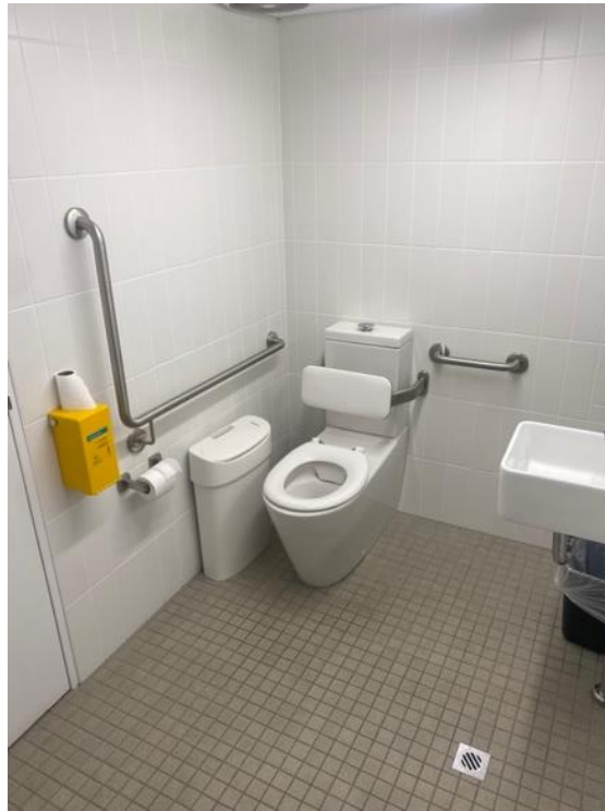
Figure 6 An image of the inside of the accessible toilet space, featuring a toilet, sink, sanitary disposal, and 2 rails either side of the toilet.
